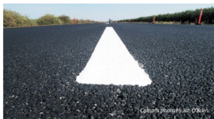
A section of new-generation road striping was recently laid on Interstate 5 near Orland, about two hours north of Sacramento.
